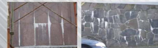
*Efflorescence on External Wall *Efflorescence on Natural Stone
