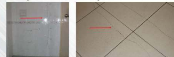
*Cracking of Wall Tiles *Cracking of Floor Tiles
